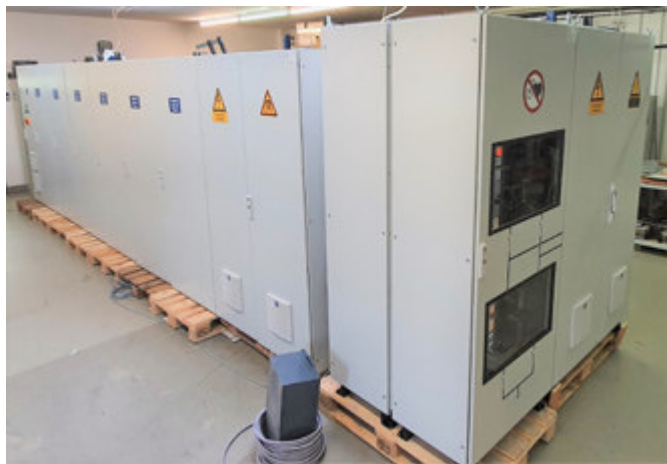
Figure 1: Not quite commonplace: the new 35kA surge current system of IPH in Berlin.
